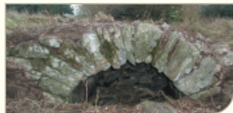
Stone bridge located over a reclamation drain in Ballinacurra (Weston). (Photo I.A.C. Ltd.)
